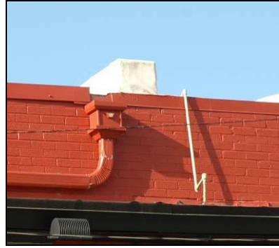
This building's mechanical equipment is inconspicuously mounted on the roof to minimize visibility from the street.
