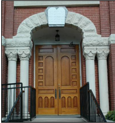
The rusticated door surround with column supports and paneled wood doors are character-defining features of this Romanesque Revival building.
