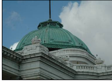
On this Classical Revival government building, the molded cornice, roof balustrades, and dome are important character-defining features.
