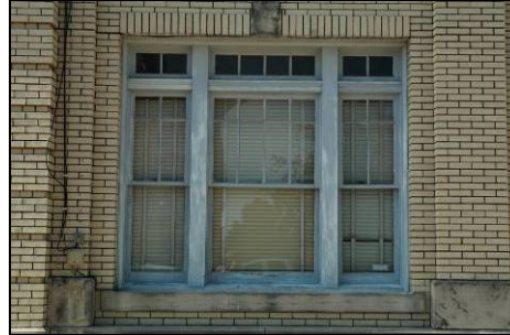
The geometric grid of muntins and number of lites in this building's double-hung windows are character-defining features.
