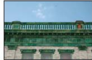
The terracotta roof parapet with balustrade and cornice is an important feature of this Italianate commercial building.
