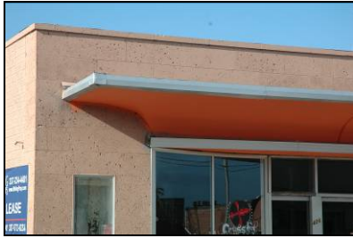
The paint color and curved edges of this cantilevered canopy are character-defining features of the building's Art Deco Style.
