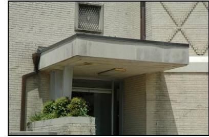
This concrete cantilevered canopy is consistent with the use of materials in this building.
